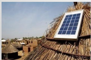
Solar Home System
